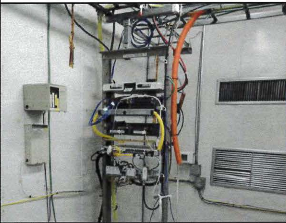
B EXISTING AUX EQUIPMENT RACK
