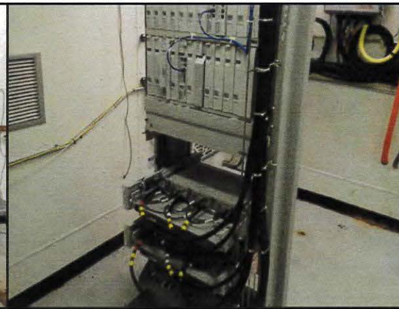
D EXISTING CDMA RACK
