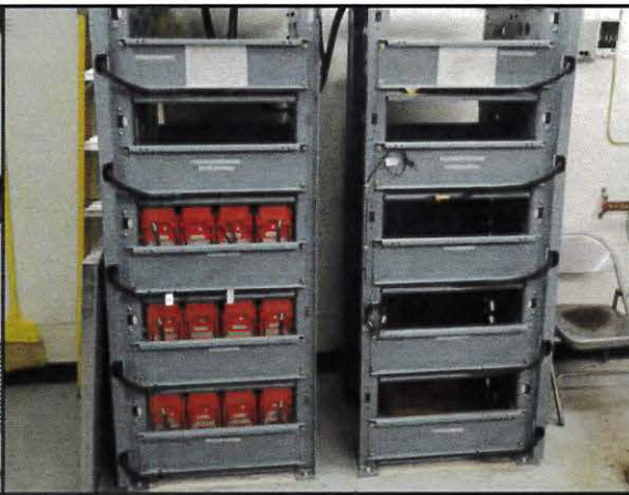
C EXISTING POWER BAY RACK
