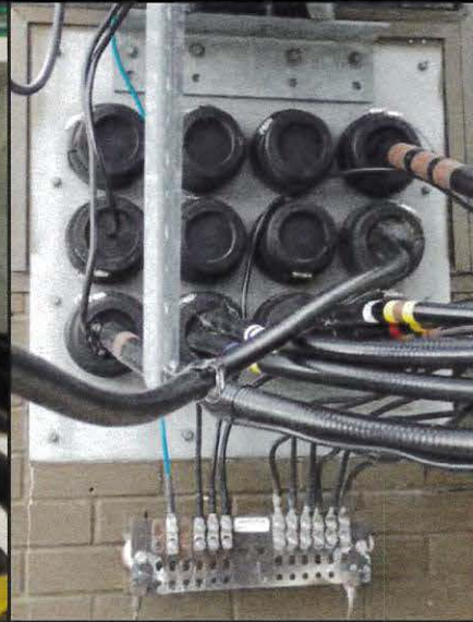
D SHELTER COAX PORT (SHELTER EXTERIOR)
