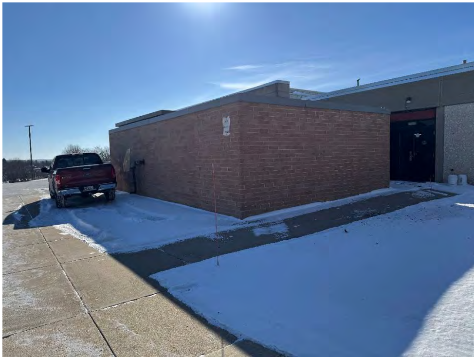
View of the fire suppression equipment room and location of former aboveground storage tank.
