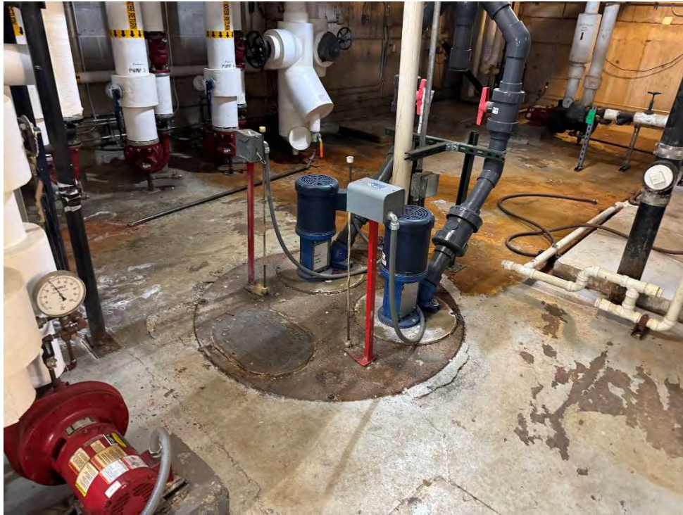
View of a sump in a mechanical room in Northview Hall.
