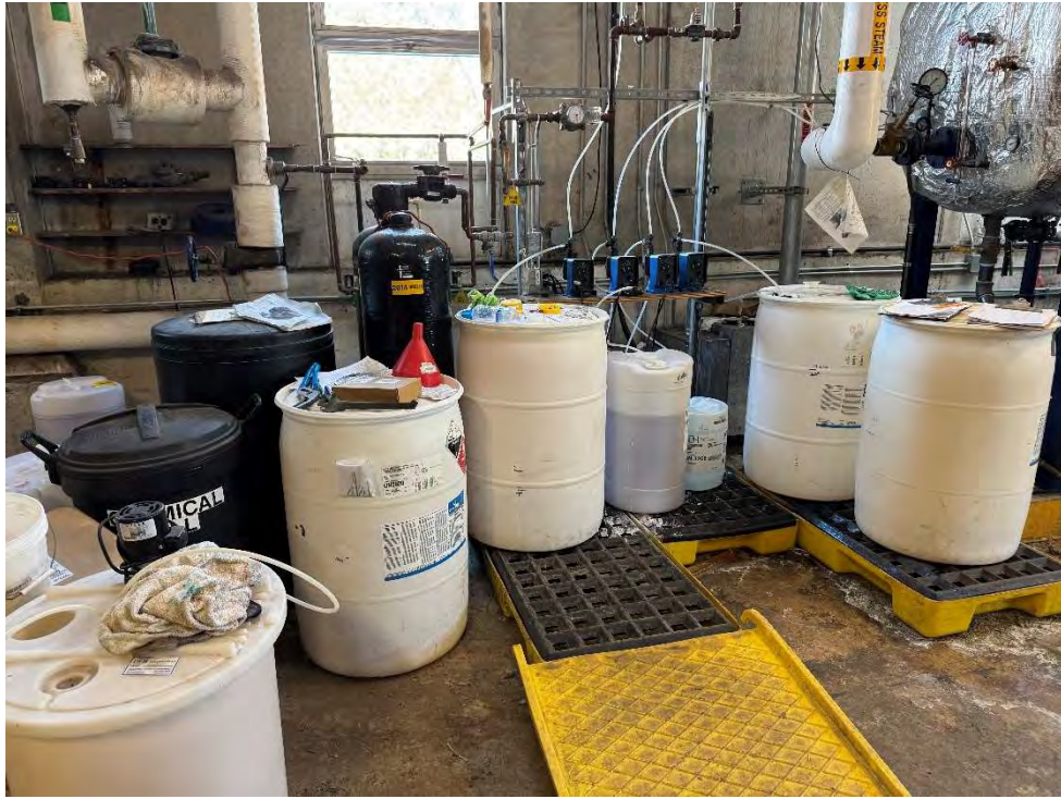
View of boiler chemicals stored in the boiler room.
