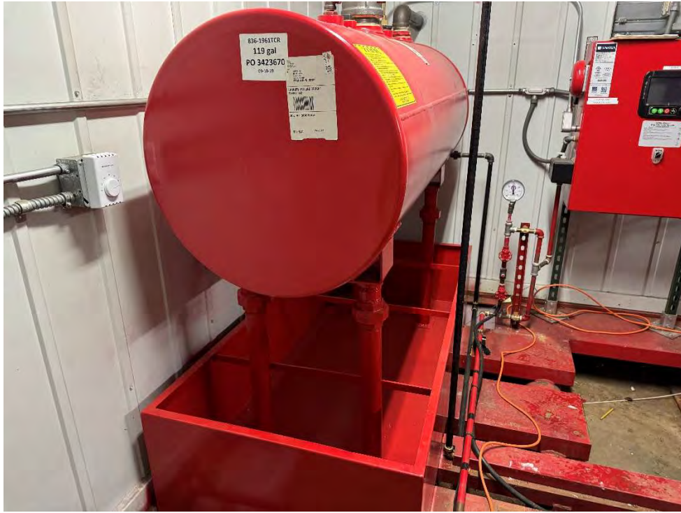
View of a diesel tank and containment dike associated with the fire suppression system.
