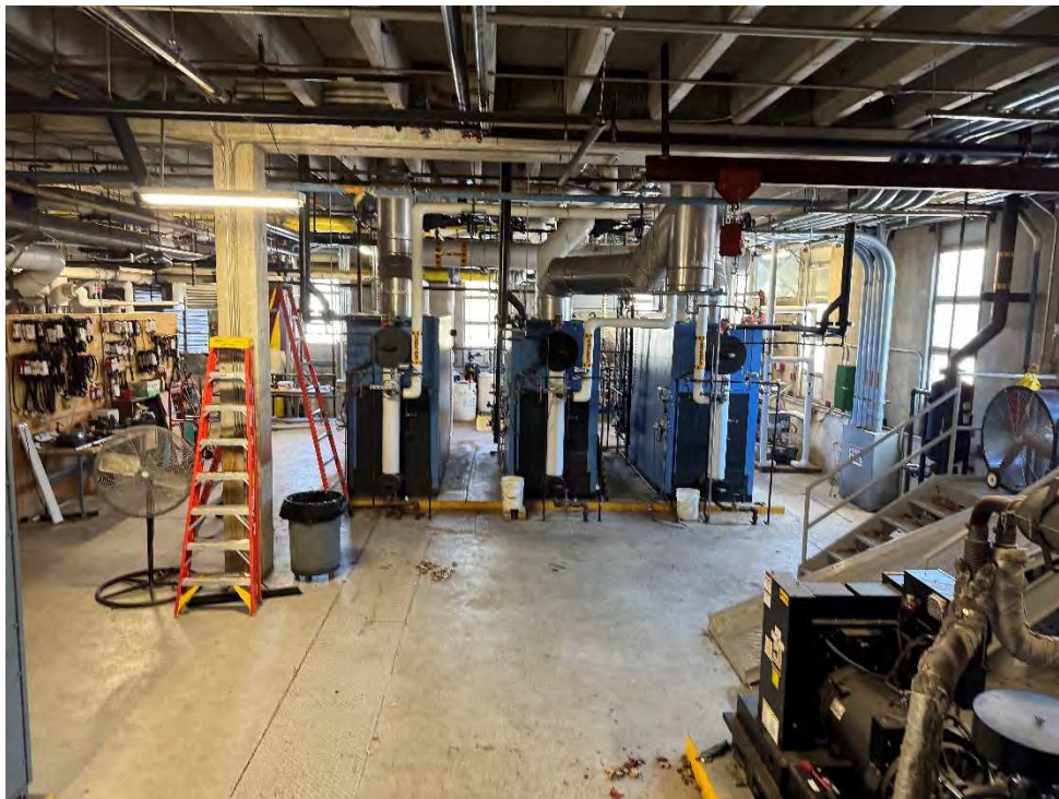
View of the boiler room in the Field House. The boilers provide steam heat to all four academic buildings.
