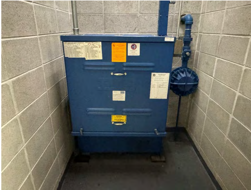
View of an elevator equipment room in Southview Hall.
